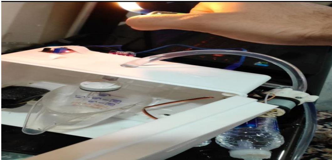
Fig. 6. Operates Water Pump When Detecting Fire.
